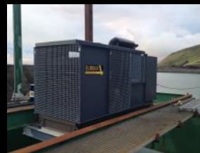
Hydraulic Power Pack
